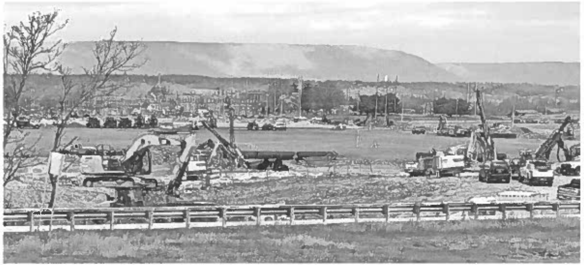
Endurance Real Estate Group, out of Radnor, is building a logistics facility just off Interstate 81 Exit 10 in Marion. PHOTOS BY AMBER SOUTH/PUBLIC OPINION
